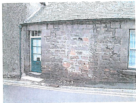
Blocked in doorway Ramsey's Street
